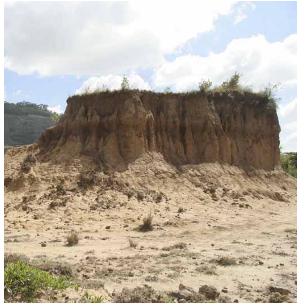
The extent of soil erosion, caused by baking sun and torrential rain, is graphically illustrated by this picture from Oromia, Ethiopia.
